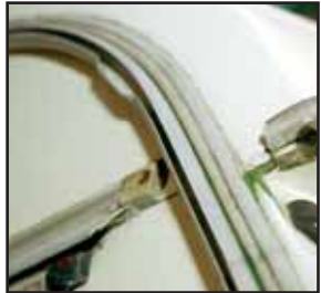
Rusting screws may mean water leaks
