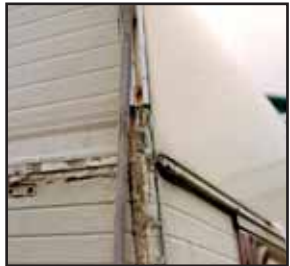
Check for failed mastic
